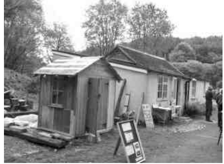
Replica Ground Frame Hut under Construction and the 1960s extension to Chelfham Station behind (Ed)
