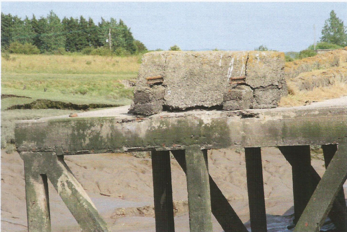
Two 2015 views of Wick St Lawrence Wharf on the WC&PR prior to raising the flood defences. The raised track bed due to subsidence is clearly visible. (Bob Edwardes)
